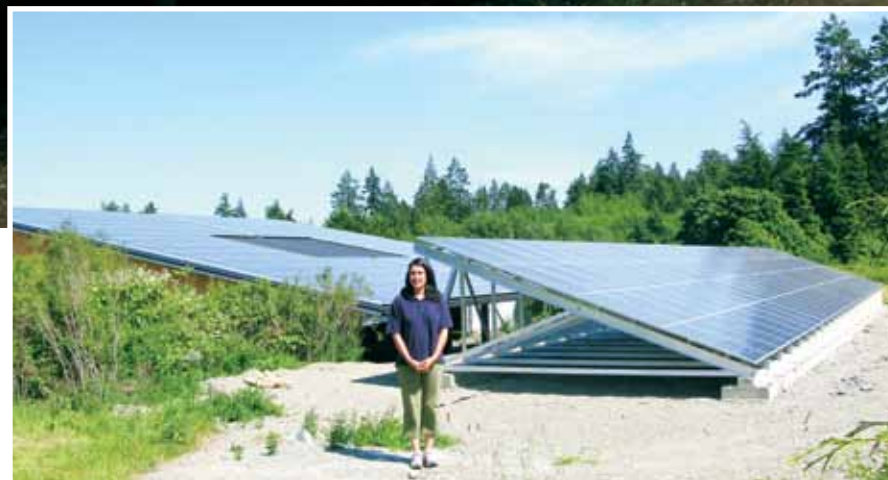
Jessica Bekker, University of Victoria Engineering Co-op student in front of 40kW and 22kW photovoltaic systems.
